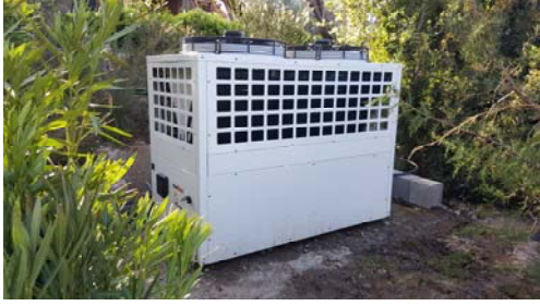
Mandarin Oriental Otel Binası-GÖLKÖY Airpool AWR72R - 38 kW
